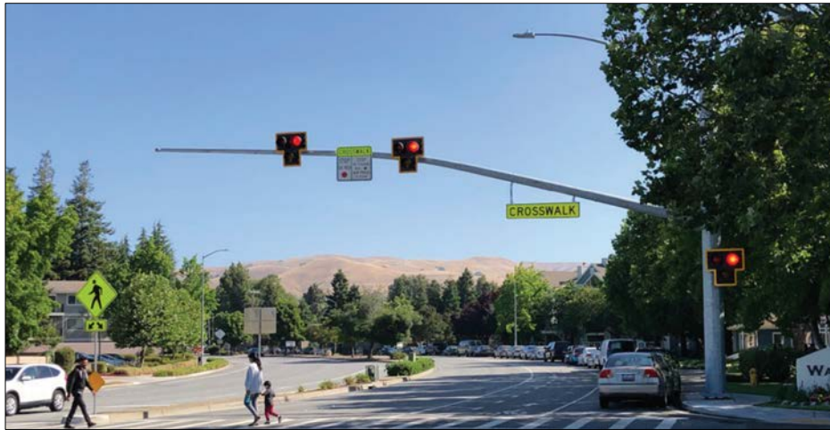
Figure 6 High-intensity activated crosswalk (HAWK) installed on Mowry Avenue at Waterside Circle in Fremont for pedestrians and bicyclists
