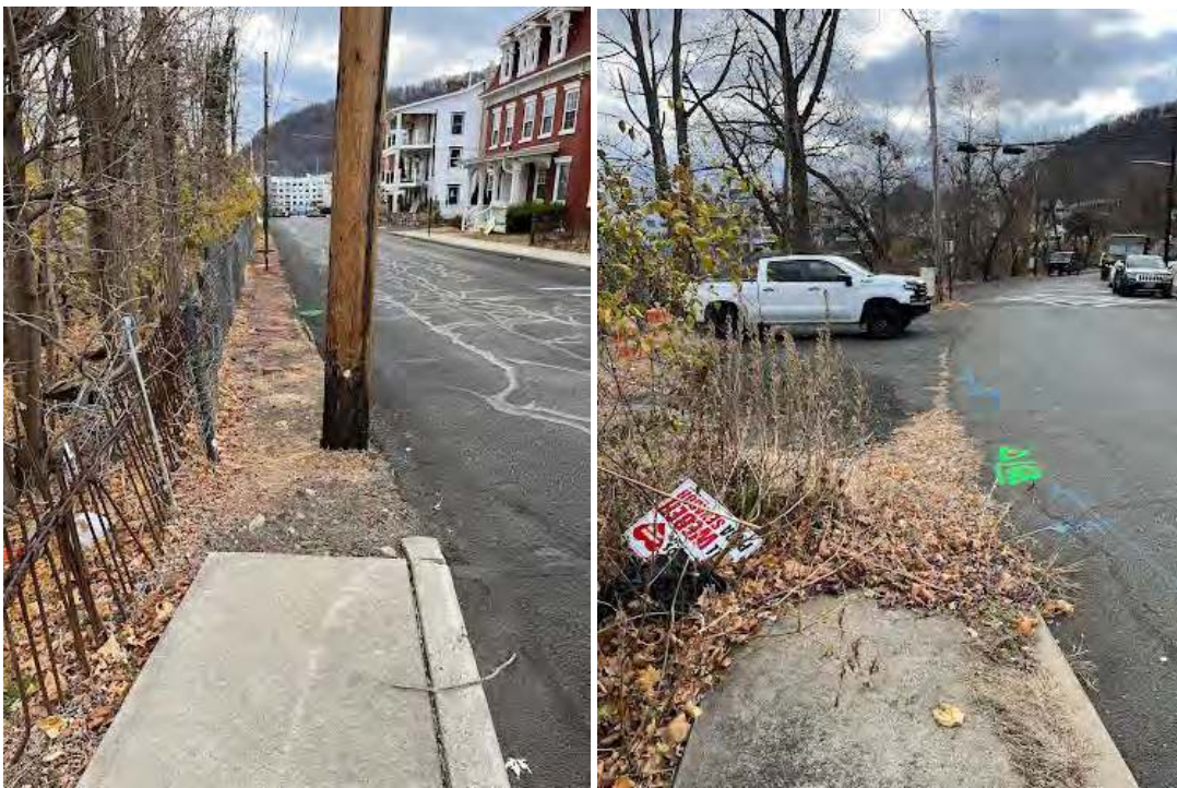
Figure 14: Missing and obstructed sidewalk conditions along First Street.
