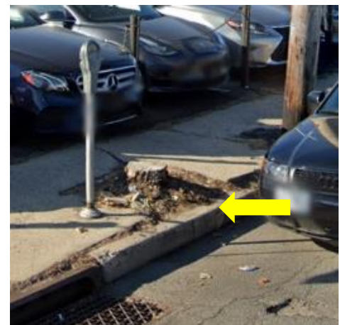
Figure 10. Poor sidewalk conditions on 417 Merrick Road causing hazardous conditions for sidewalk users. Source: Google.
