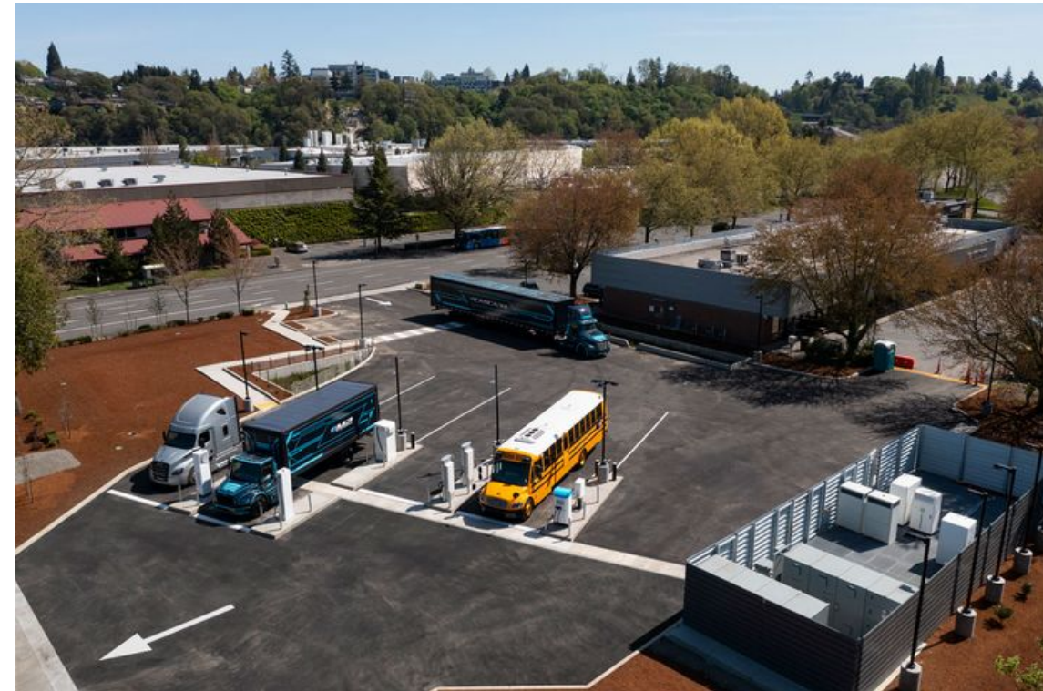
Electric Island Heavy Duty Vehicle Charging Station, Portland, Oregon
