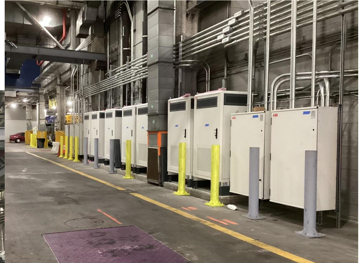
Grand Ave – Power Cabinets
